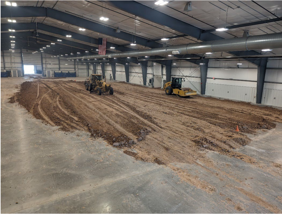
1,500 tons of dirt will fill the main event floor at the Event Center at Archer to create an indoor dirt arena.
